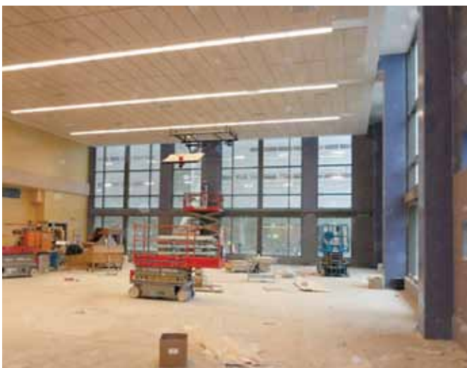
The new two-storey gymnasium is under construction in this photo, taken in February 2012.
